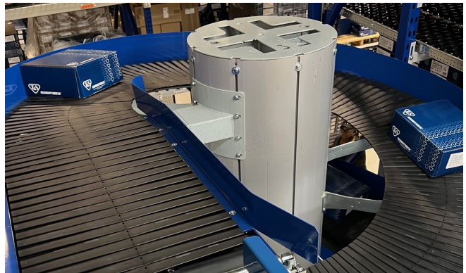
The installation includes four spiral turns that deliver material to ground level.
