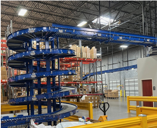
A motor-driven roller (MDR) spiral turn lifts packages to an overhead conveyor that delivers them to shipping.
